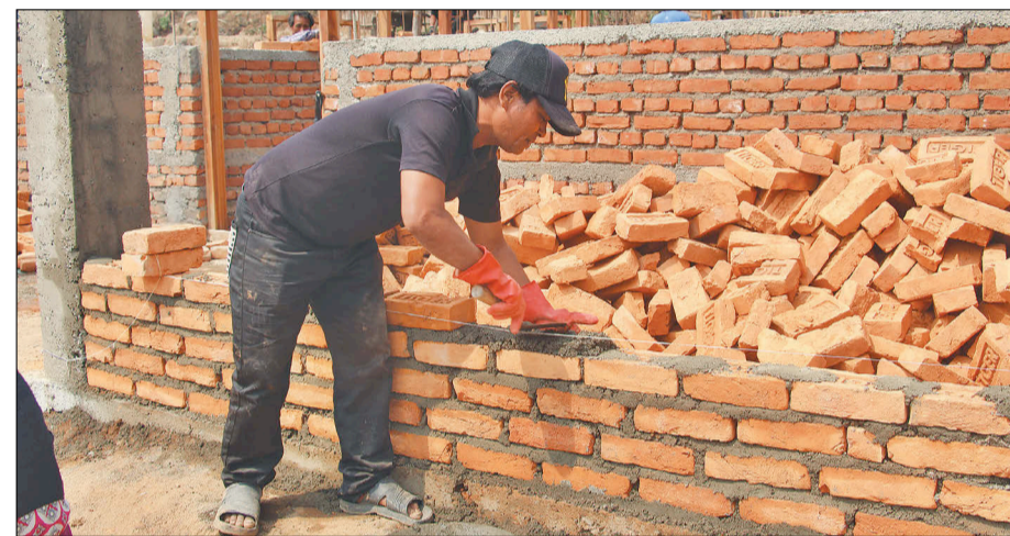
A bricklayer builds a house wall at Bhimpheedi Rural Municipality in Makwanpur.
