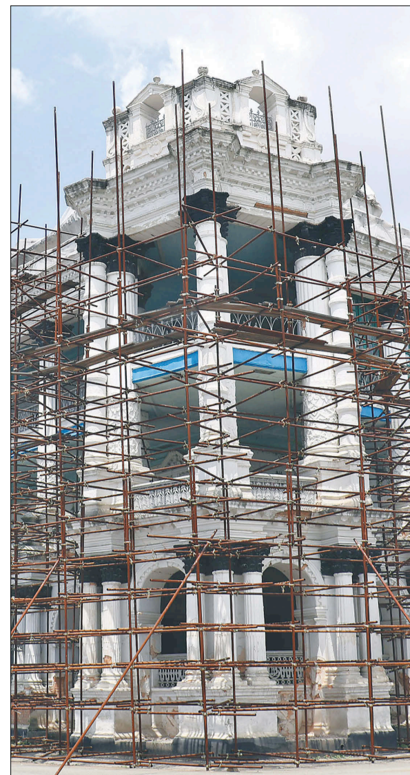
Retrofitting work on Singha Durbar begins on Wednesday with the installation of scaffolding around the building damaged by the earthquake on April 25, 2015.
