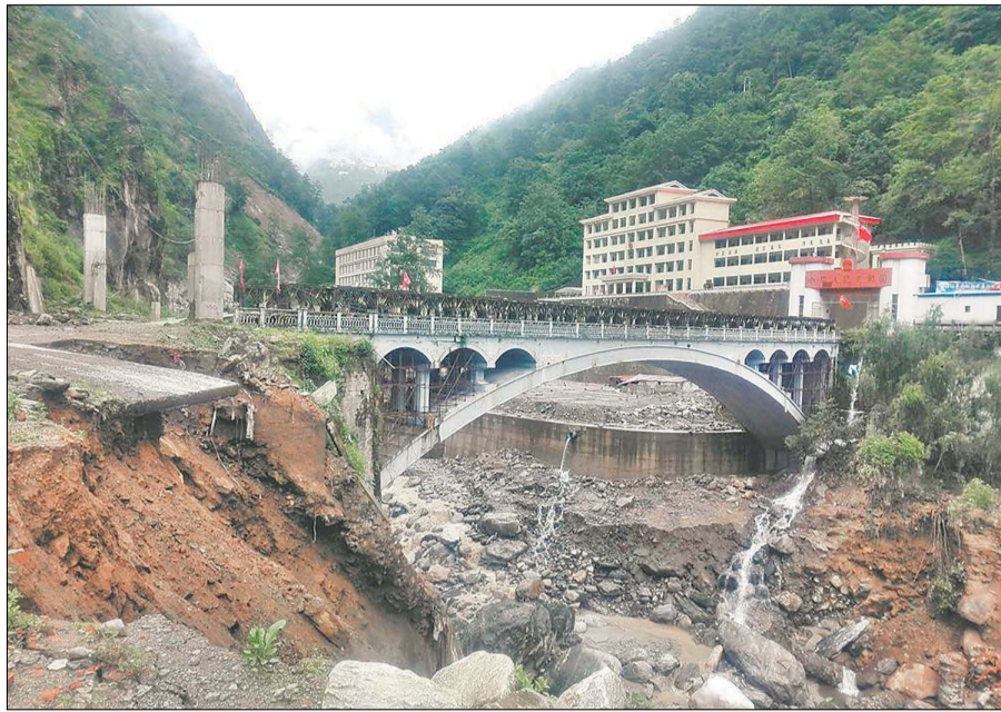
■ The Nepal-China Friendship Bridge of Tatopani, Sindhupalchok, following the 2016 flood. POST FILE PHOTO
