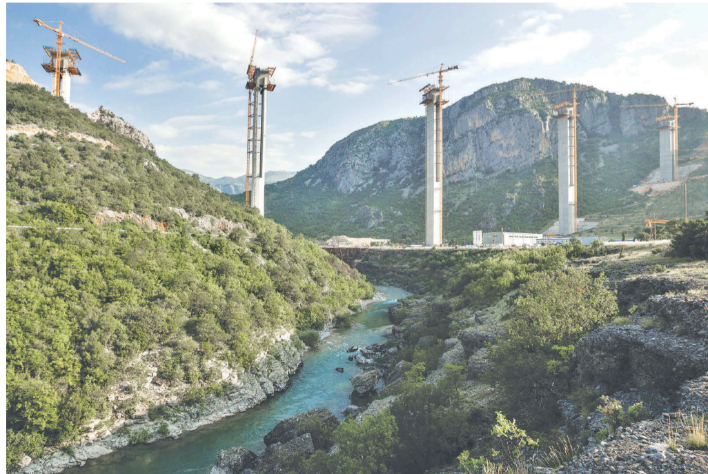
Cement pillars above Moraca river canyon are seen at a bridge construction site of the Bar-Boljare highway in Biocce, Montenegro.
