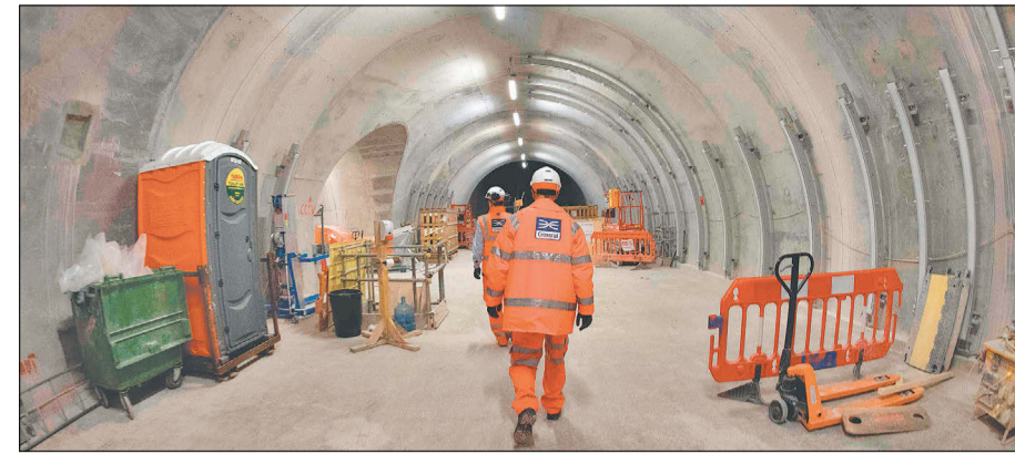
■ Workers walk through a tunnel during construction on the platform level of the new Crossrail section of Farringdon Station in London. London's new train line, which was set to open through the city centre in December, has been put back for nearly a year.
