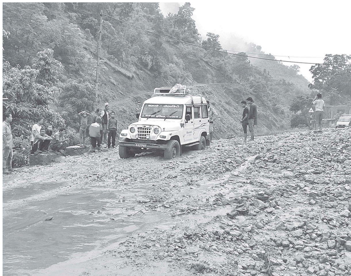
A section of the Gwalichaur-Jaljala-Ranasinkiteni road has been damaged because of the rains in Badigad.
