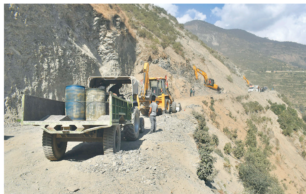
Workers construct a road section at Chainpur, Taklakot in Bajhang. The road that will connect China is expected to be completed within the next two years.
