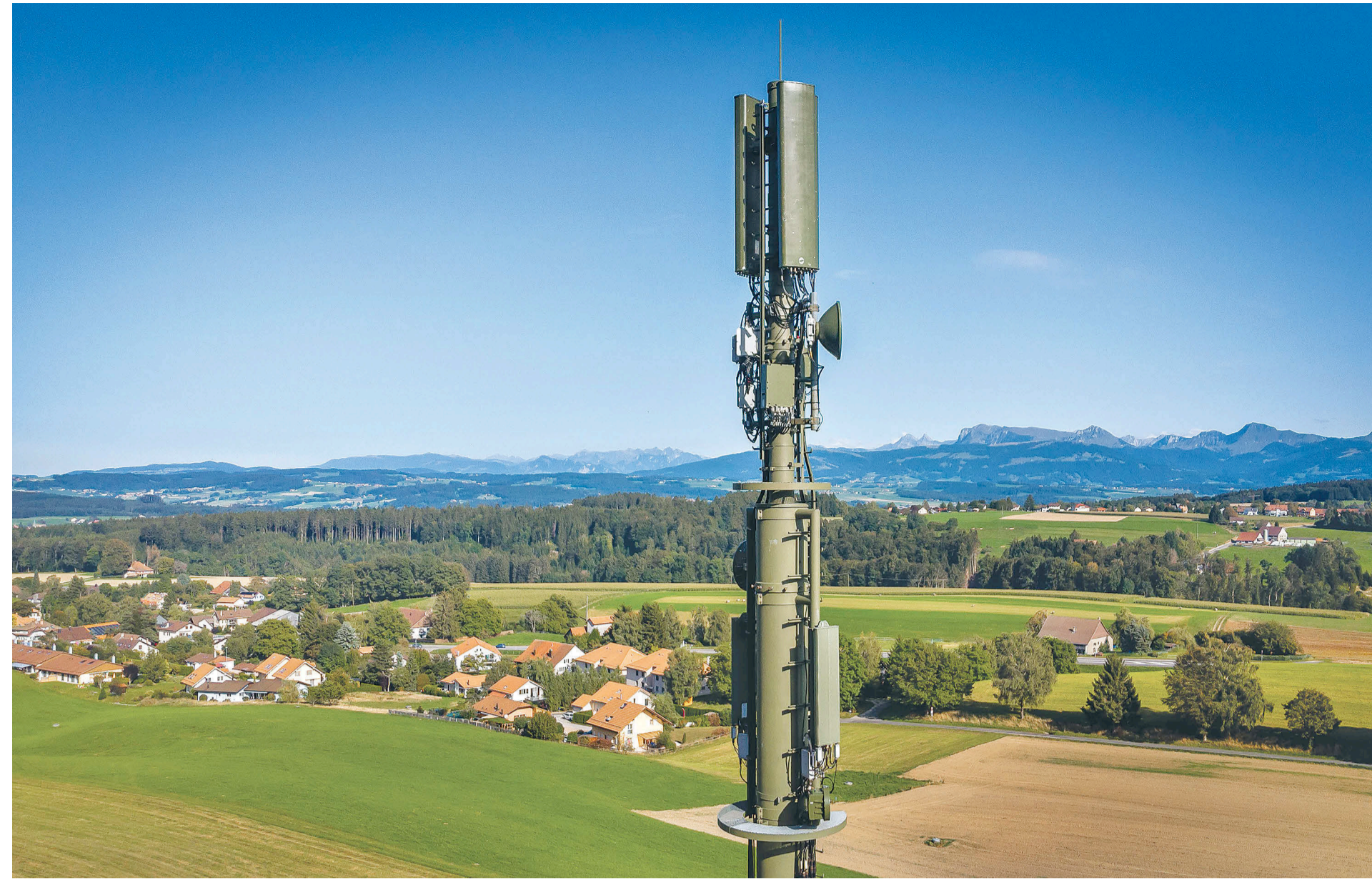
A high-speed 5G mobile network antenna is pictured near Montpreveyres, western Switzerland, on Sunday. Switzerland was among the first countries to begin deploying 5G, but health fears over radiation from the antennas that carry the next-generation mobile technology has sparked a nation-wide revolt.
