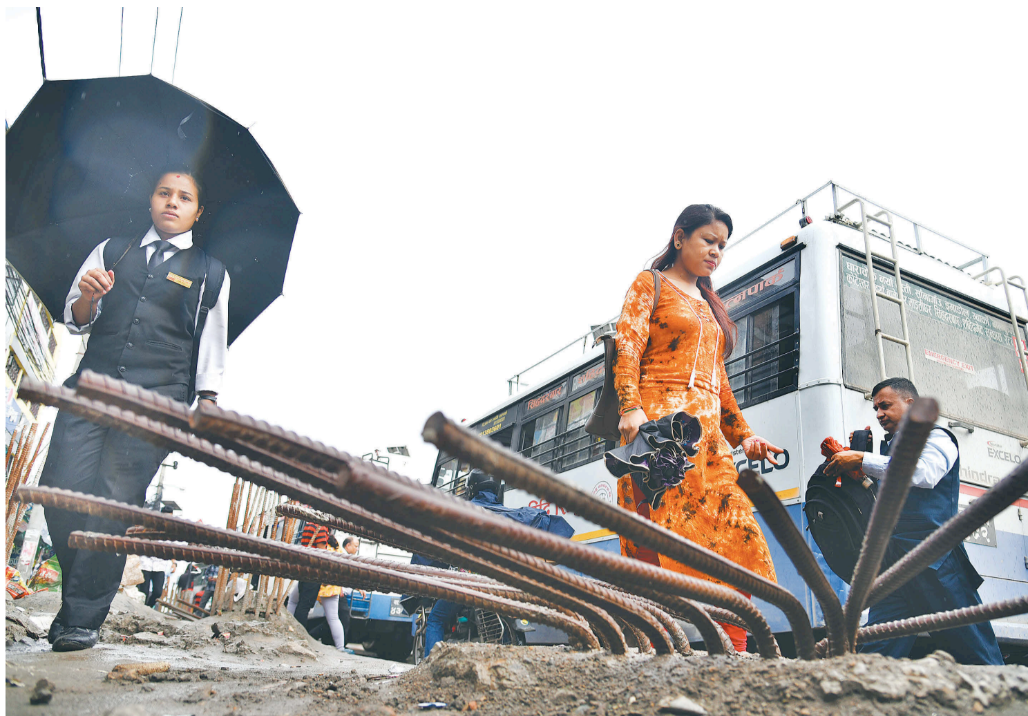
Steel rods jut out on a roadside, posing injury risk for pedestrians in New Baneshwor, Kathmandu.
