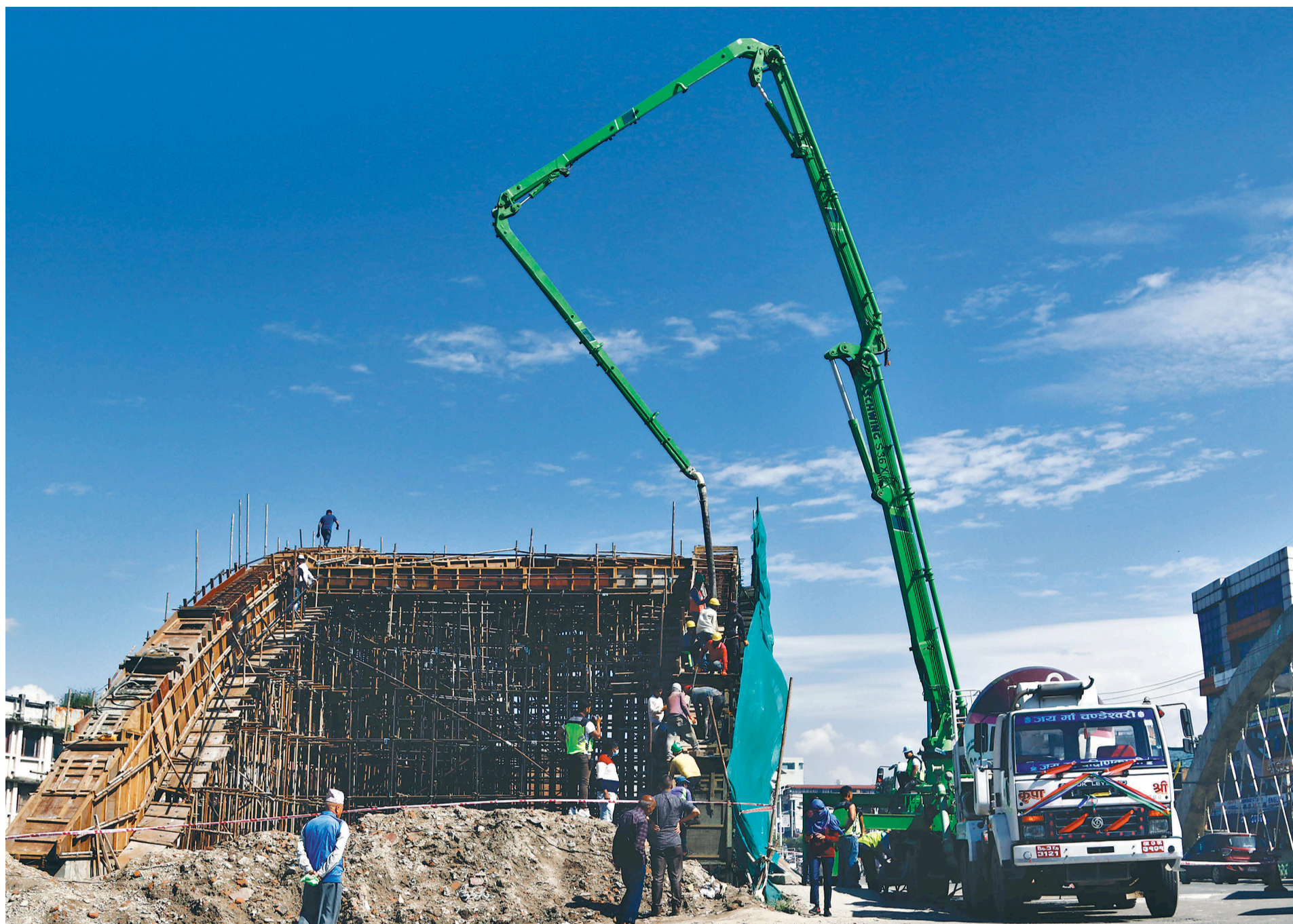
Workers construct an arc bridge over Dhobikhola near Bijuli Bazaar with the help of a transit mixer machine on Friday.
