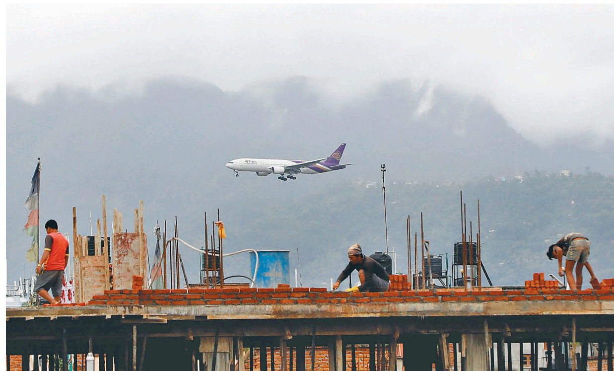
Builders work on an under-construction building while a Thai Airways aeroplane flies in the background in Lalitpur on Saturday.
