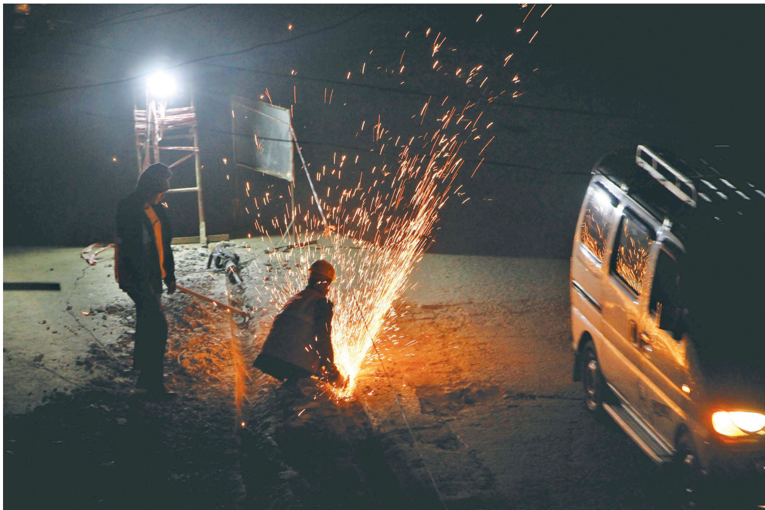
Workers at the Melamchi pipeline installation site in Nayabazar, Kirtipur, on Monday.
