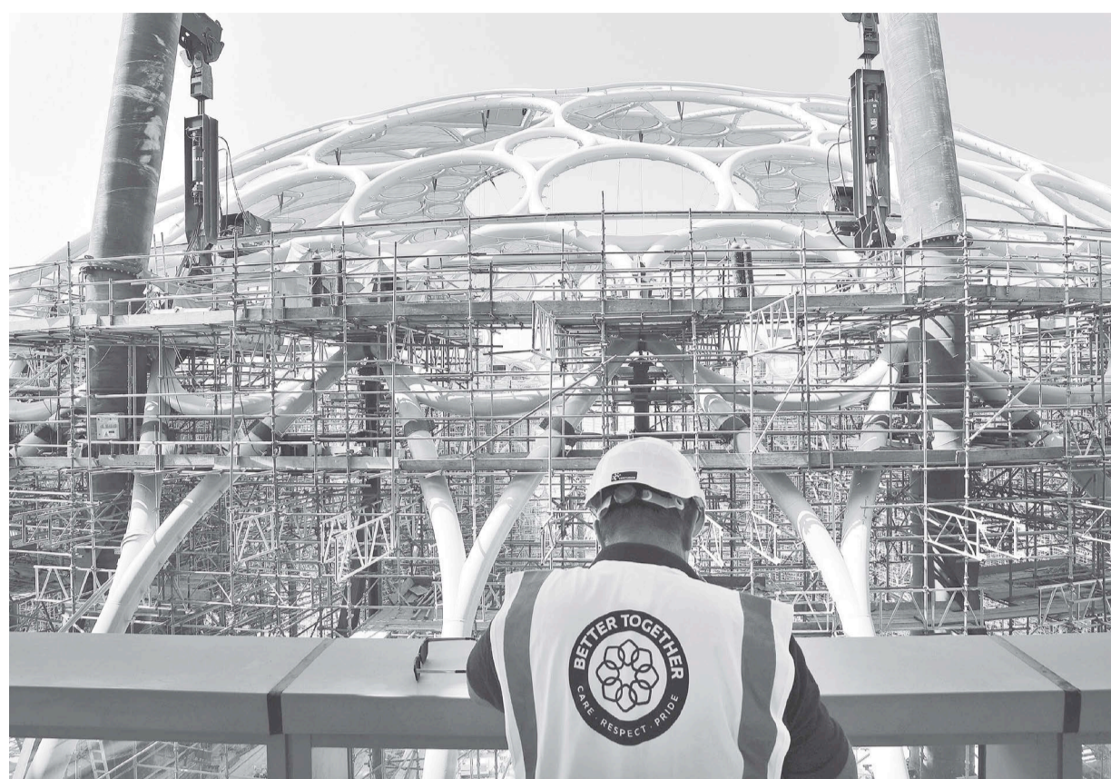
An employee of the Dubai Expo 2020 visits the Al Wasl Dome at the under construction site of the Expo 2020 in Dubai, United Arab Emirates.
