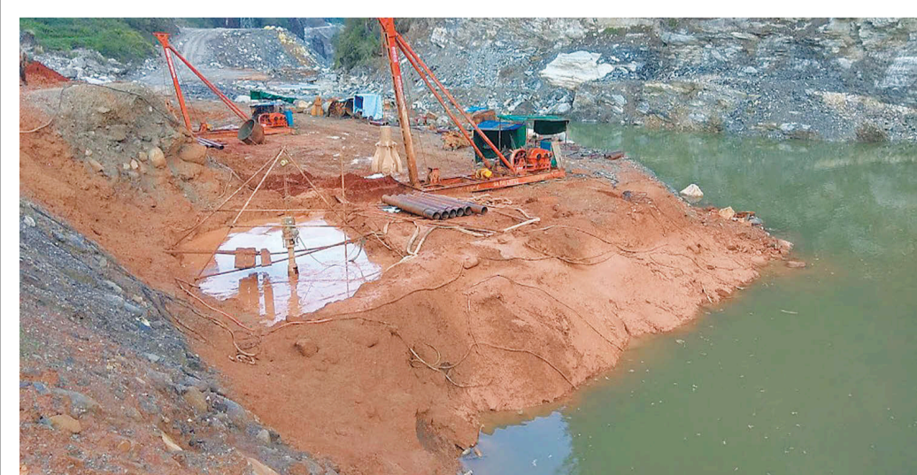
A general view of the Middle Bhotekoshi Hydroelectric Project construction site in Sindhupalchok district.
