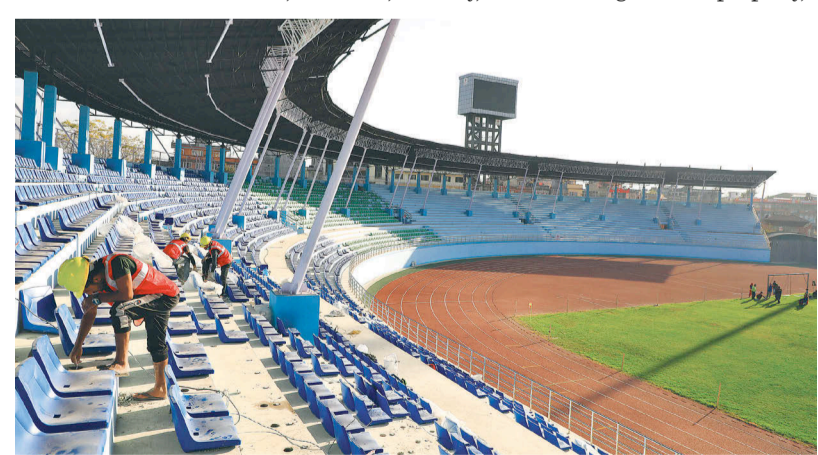
Construction of Dashrath Stadium, the main event venue, was rushed at the last minute. POST PHOTO: HEMANTA SHRESTHA
