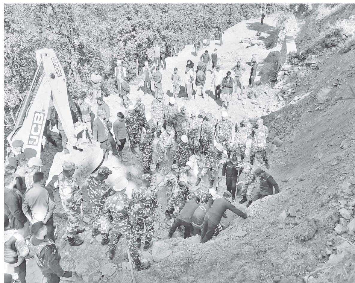
Workers were constructing a retaining wall along the Manipal-Sikles-Manang road section in Mauja when the landslide swept away the wall, burying them at around 8:05 am on Sunday.
