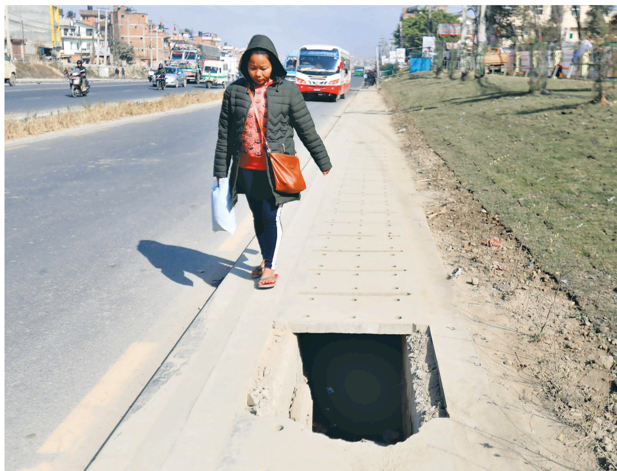
A woman avoids a broken drain cover as she walks along the footpath in Satdobato, Lalitpur.
