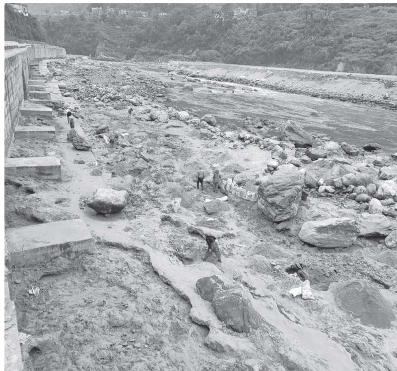
The construction of the embankment started in the wake of the devastating floods in 2013.
