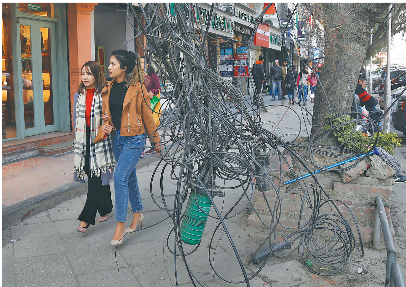
People walk past a mess of tangled utility cables at Durbar marg in Kathmandu on Friday.
