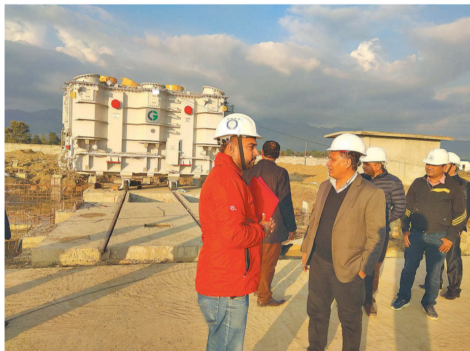
Nepal Electricity Authority and project officials at the site of under-construction substation in Nawalparasi.
