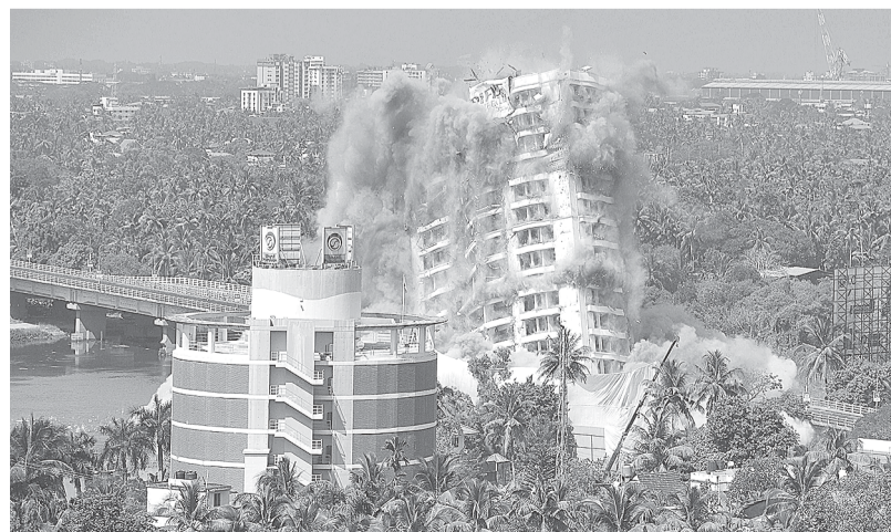
An apartment complex is pictured during a controlled implosion ordered by the Supreme Court for violating coastal construction regulations in Kochi on Saturday.
