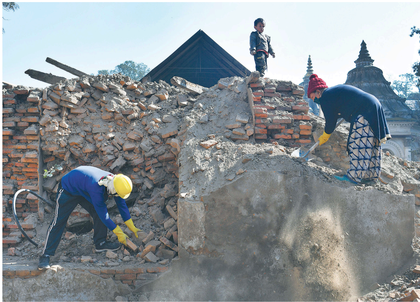
A woman joins in clearing the debris of an earthquake-damaged monument as her child watches at Guheshwori in Kathmandu on Sunday.
