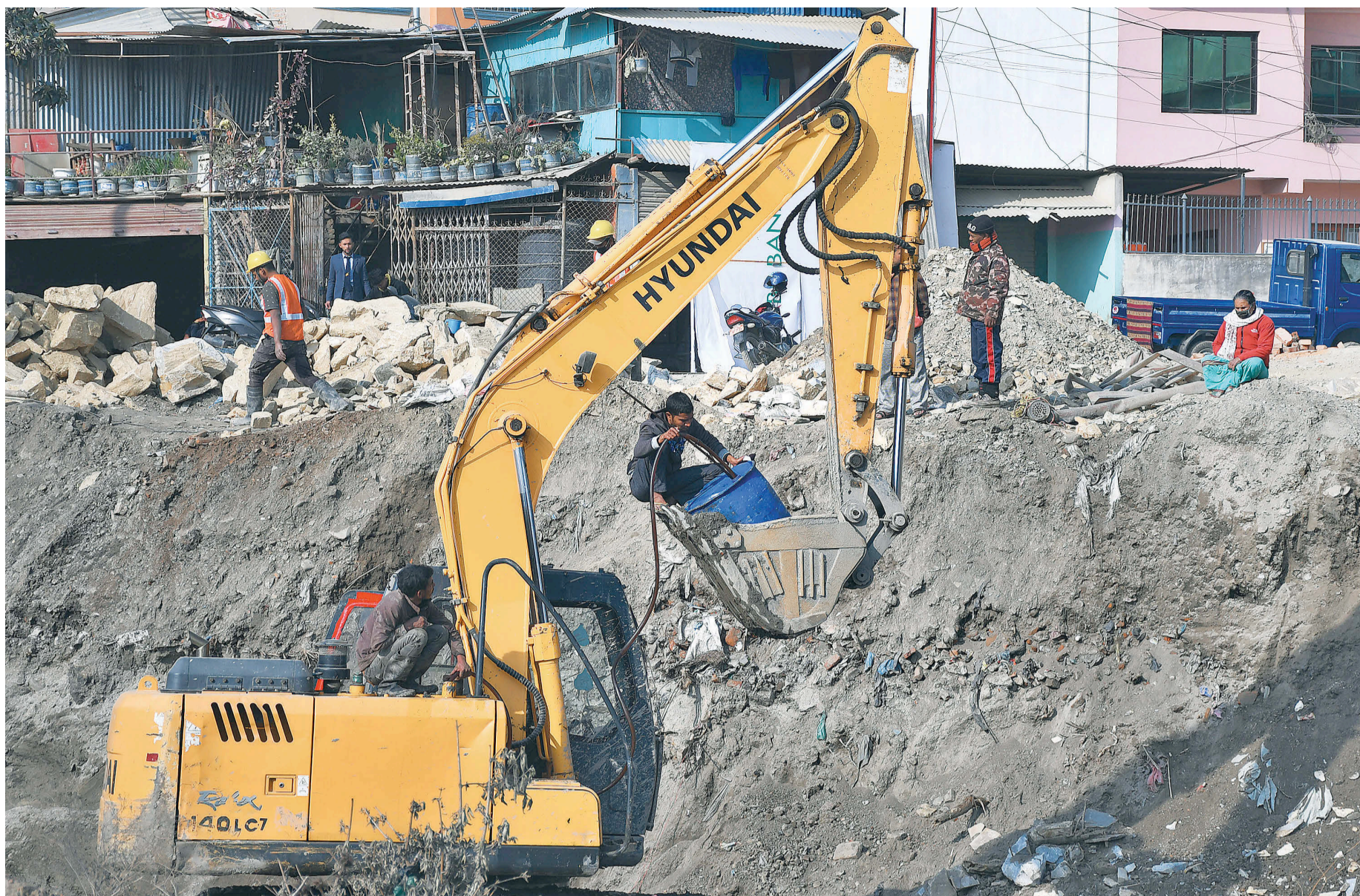
A worker fuels an excavator at a construction site in Chyasal, Lalitpur.
