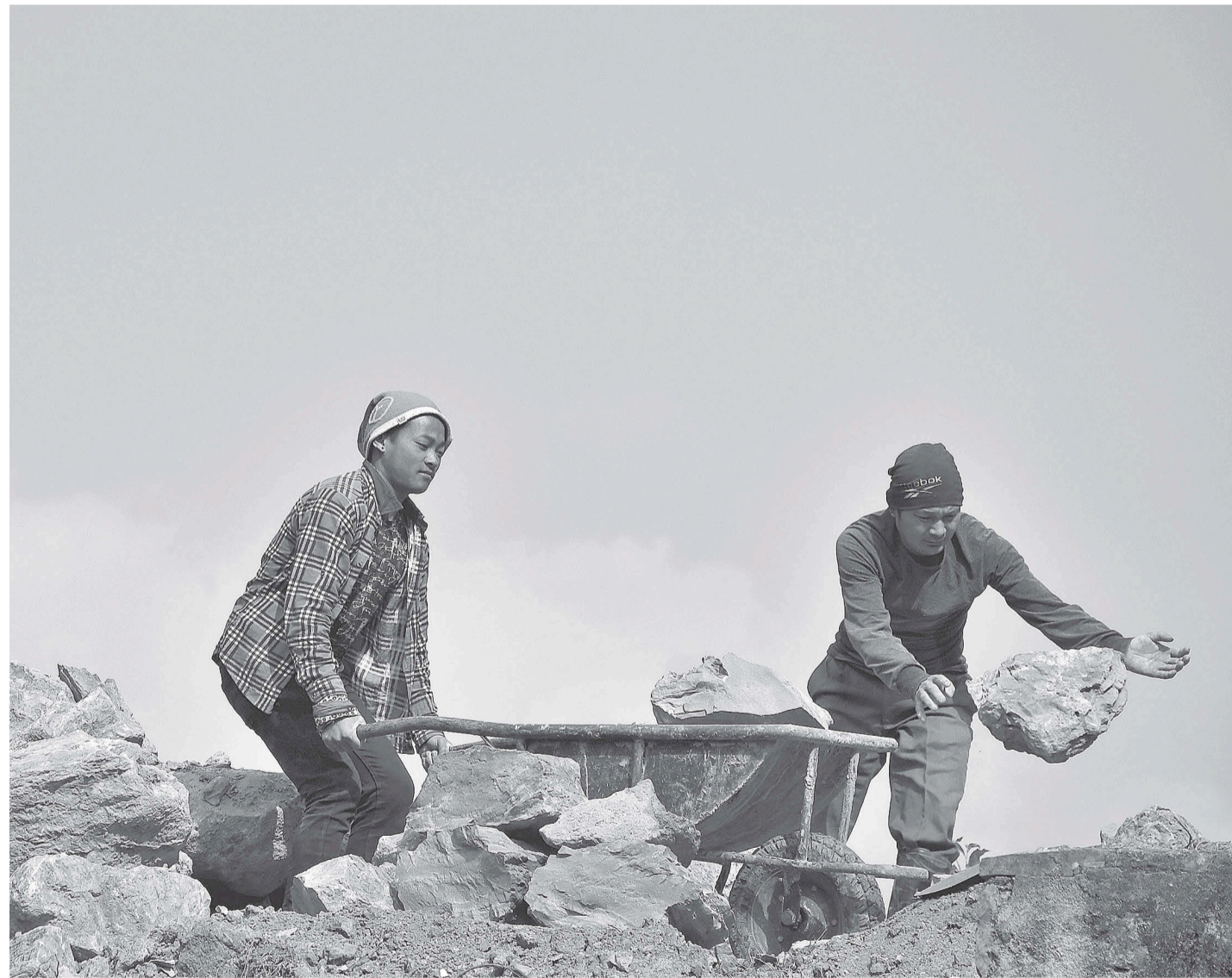
Workers arrange stones for the construction of a retaining wall along a road in Charghare, Lalitpur.
