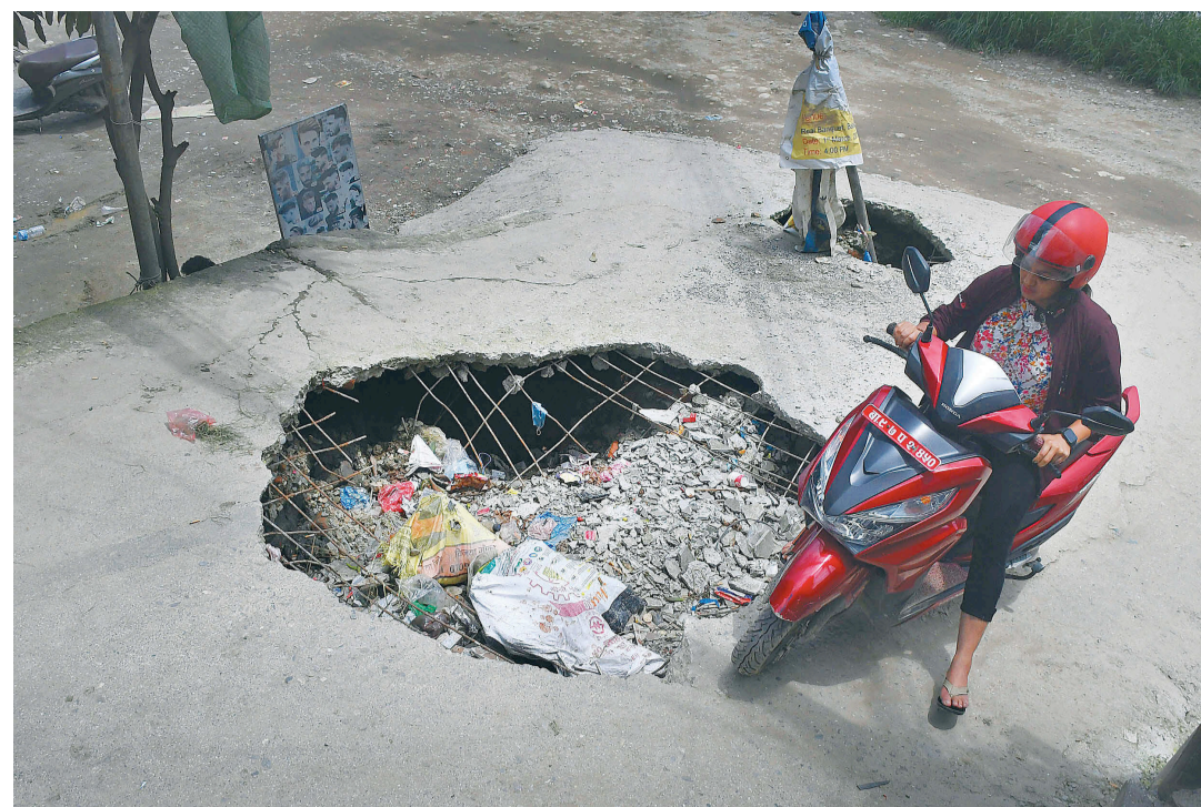
A woman rides her scooter through a damaged road section in Kalanki, Kathmandu. According to locals, the road was damaged more than a month ago, but the concerned authorities have not taken an initiative to fix it.
