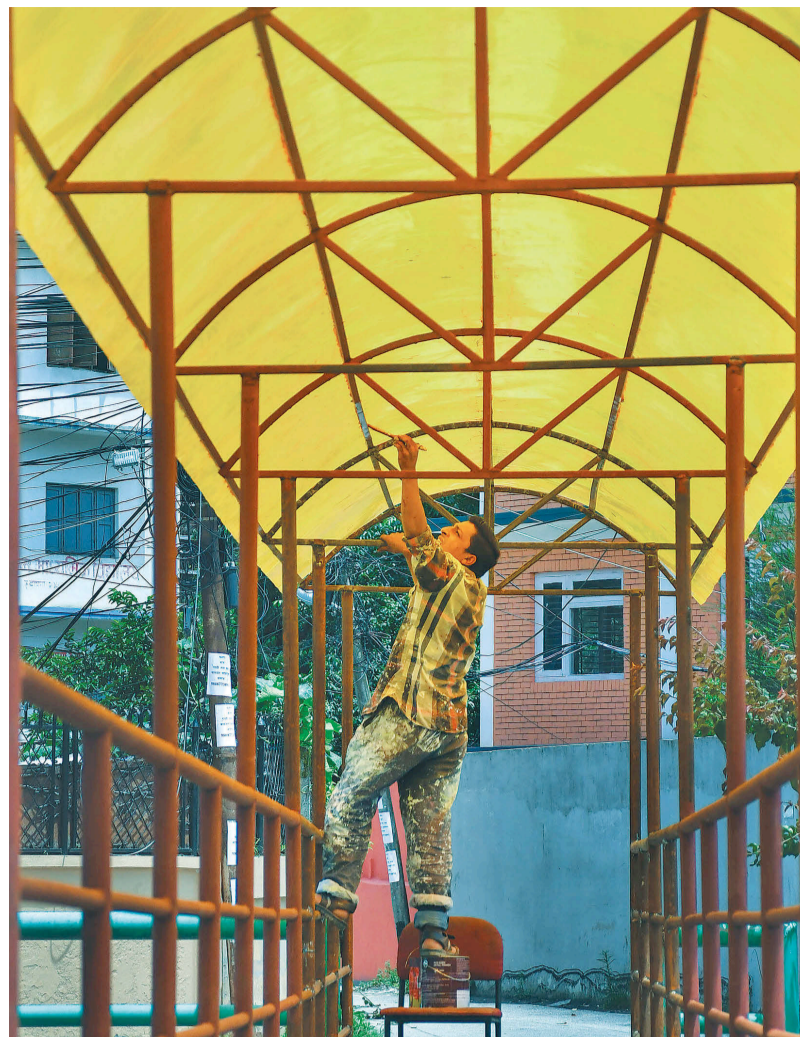
A worker applies a paint on the truss of a newly constructed footbridge over Dhobi Khola in Babarmahal, Kathmandu.
