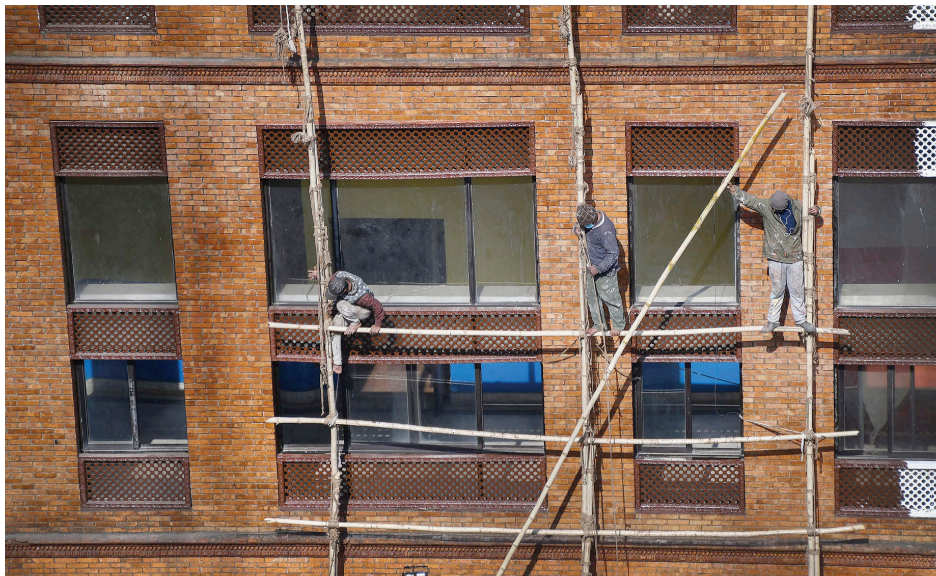
Workers with minimal safety gear disassemble bamboo scaffolding after painting a building at Jamal, Kathmandu.
