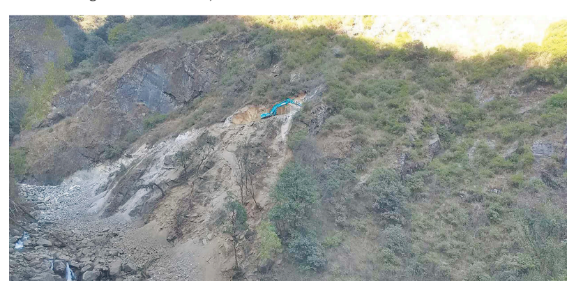
The contractor has opened 29 kilometres of the 34 km road track so far.
