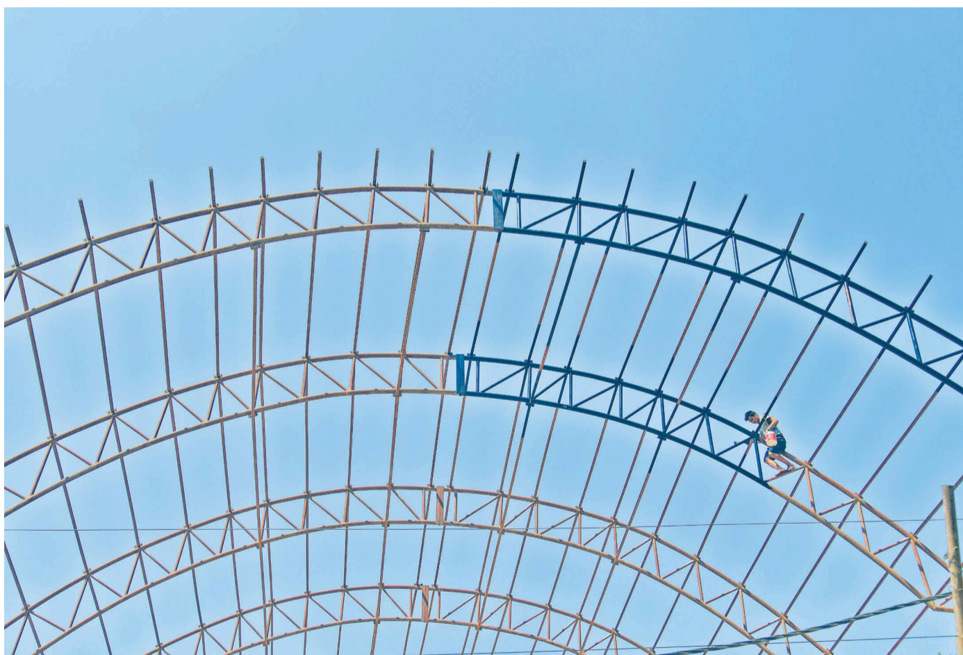
A labour paints a roof truss without employing any safety measures at Gokarna on Wednesday.
