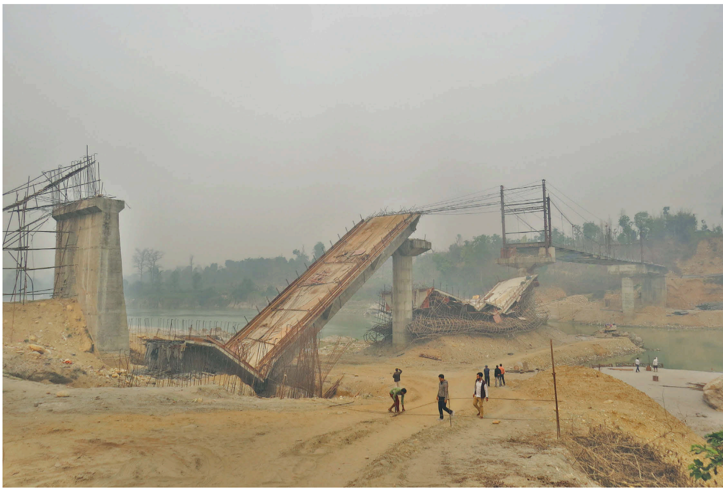
An under-construction bridge over Trishuli river in Thimura, Chitwan that collapsed on Tuesday morning.
