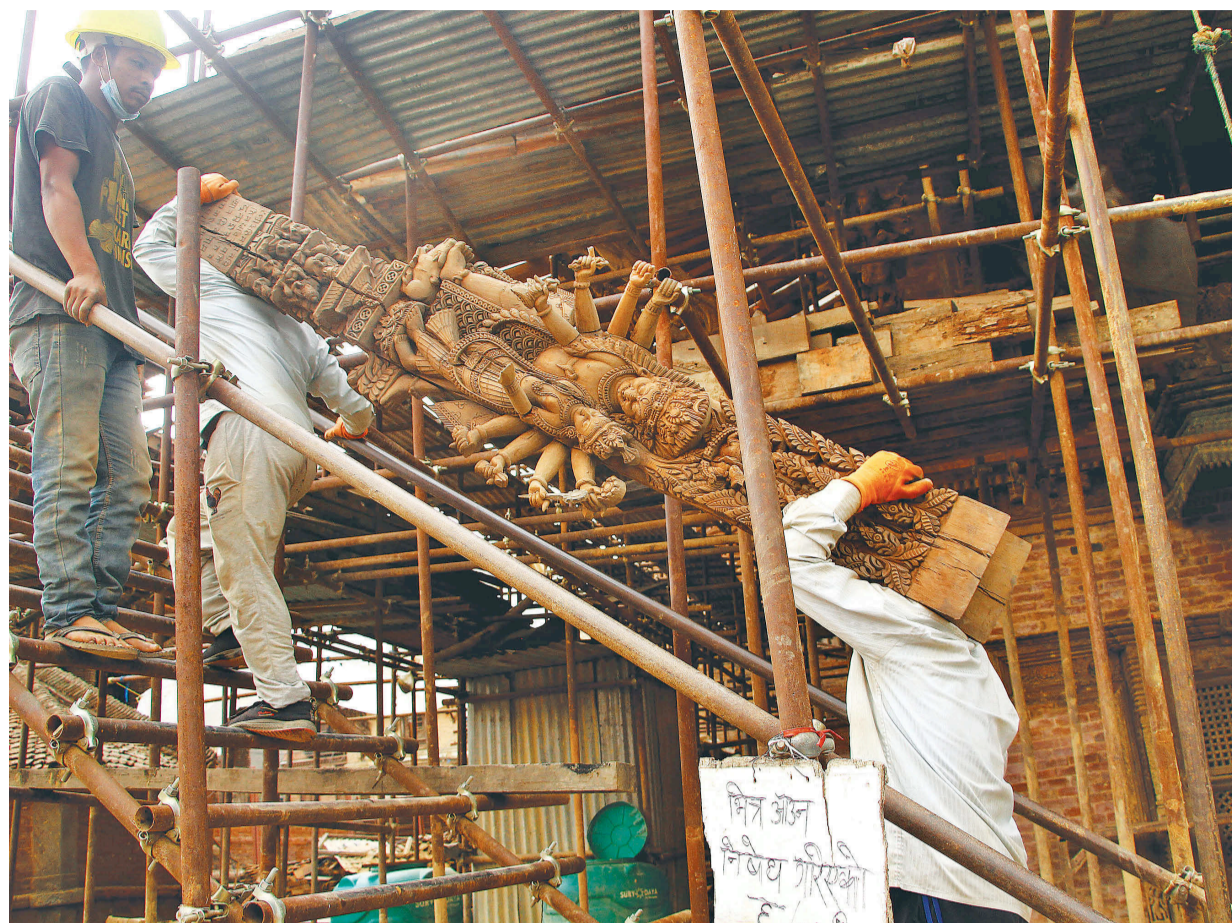
Workers carry a beautifully carved strut to be installed at the under-construction Bhimsen temple at Mangalbazaar, Lalitpur. Restoration work at the structure damaged in the 2015 earthquakes has been going on despite the restrictions imposed to curb the spread of coronavirus infections in the Valley.
