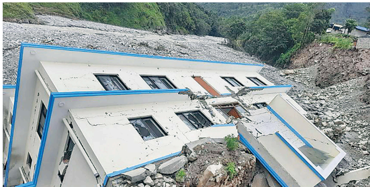
The destroyed office building of Area Police Office Helambu.
