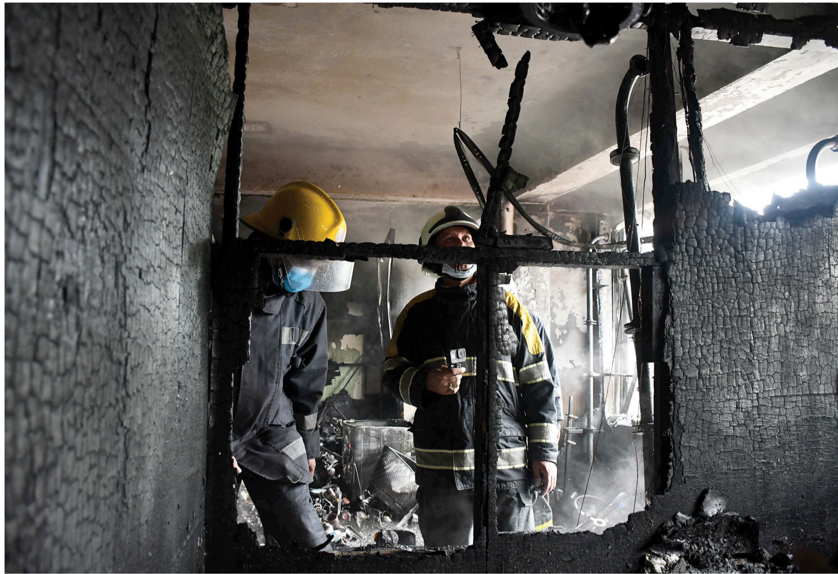
Firefighters inspect a building at Teku, Kathmandu that had caught fire on Monday.
