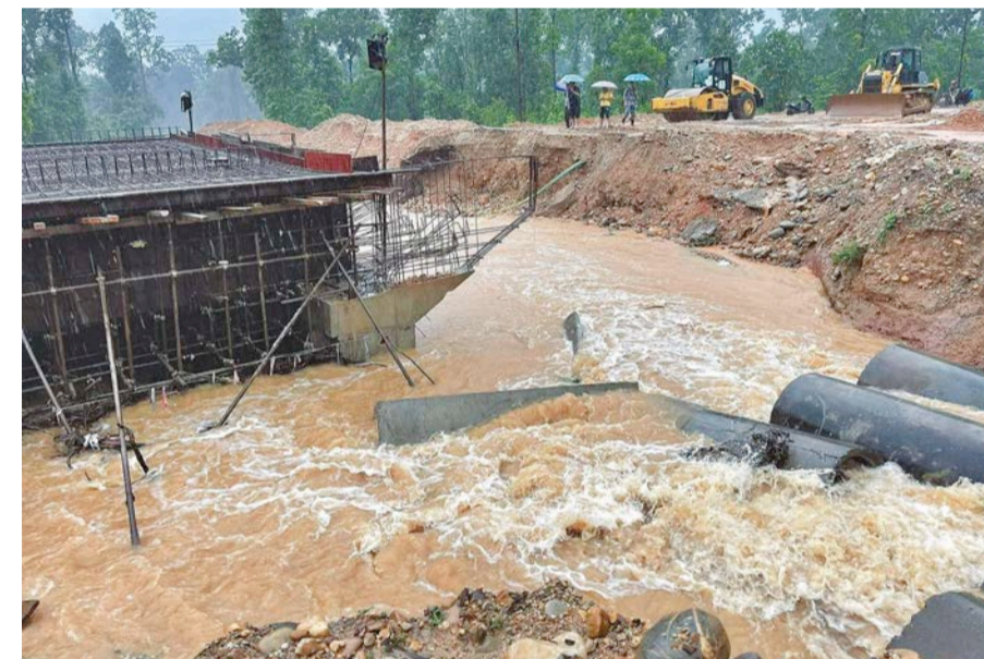
Flooded streams have swept away road diversions in three different places along the highway.
