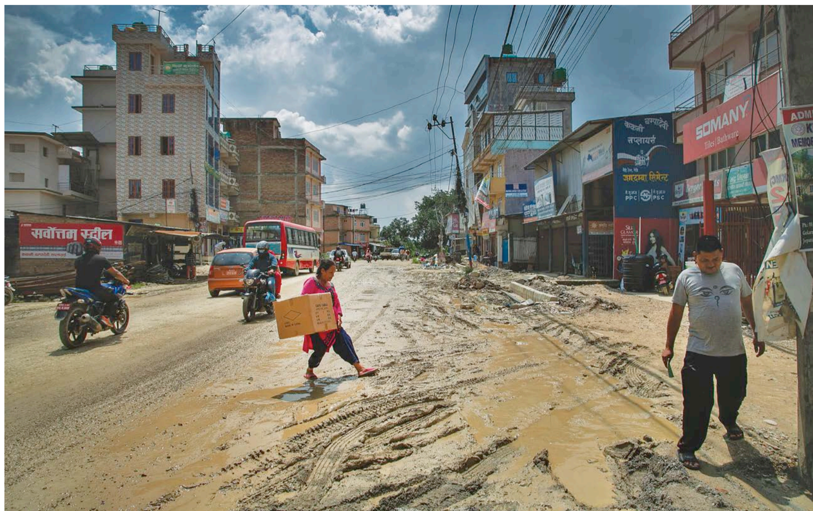
The muddied Thali section of the Chabahil-Jorpati-Sankhu road in Kathmandu earlier this week. Seven years into construction, the stretch is still full of potholes, dust and mud. POST PHOTO: PRAKASH CHANDRA TIMILSENA
