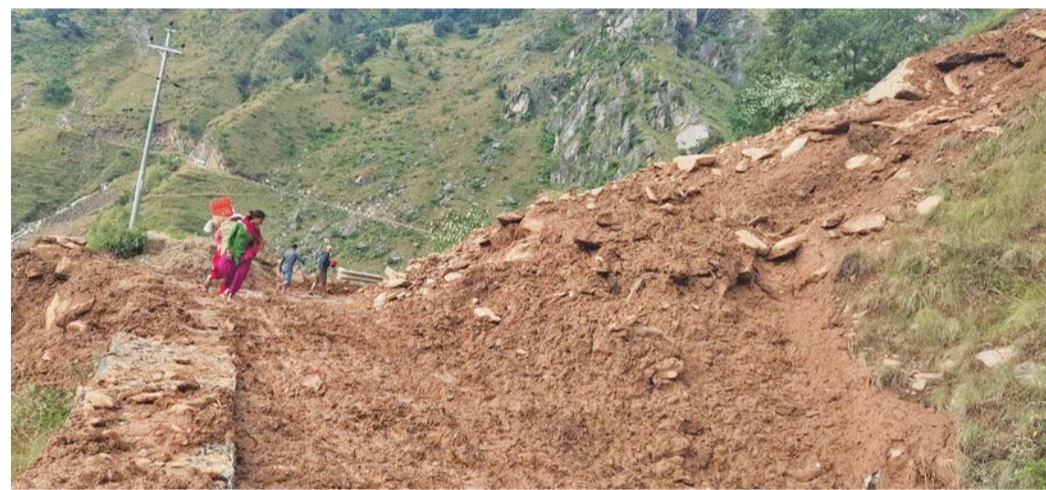
Travellers are seen picking their way through a landslide-hit section of the Karnali Highway in Kalikot this week.
