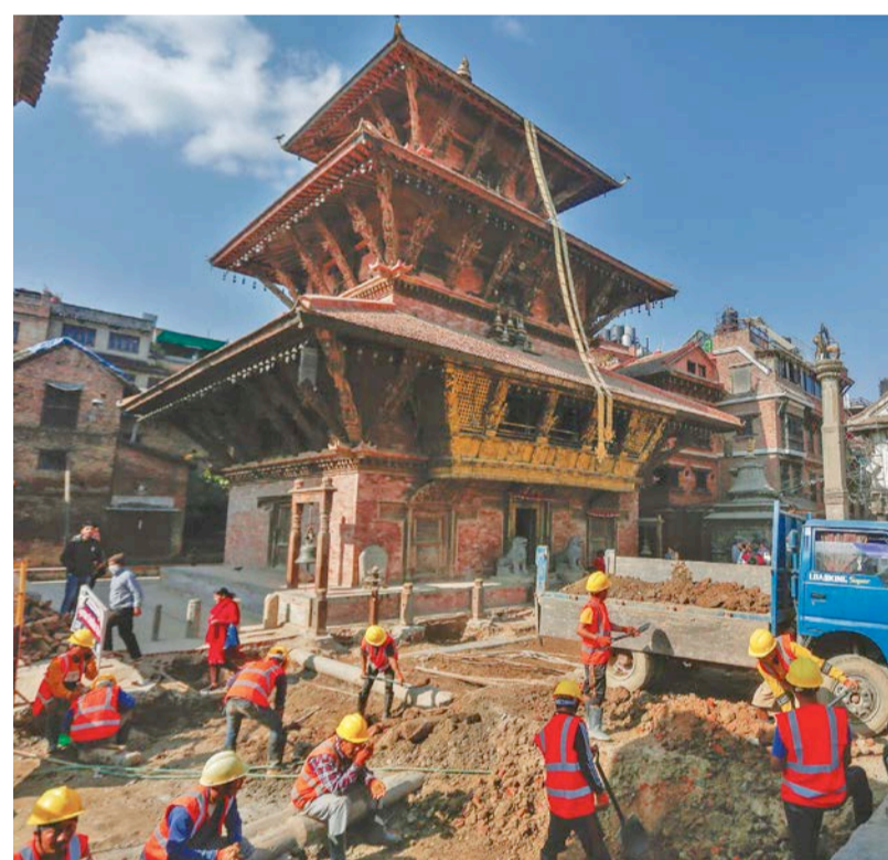
Workers load mud onto a truck at a construction site at Patan Durbar Square on Thursday.
