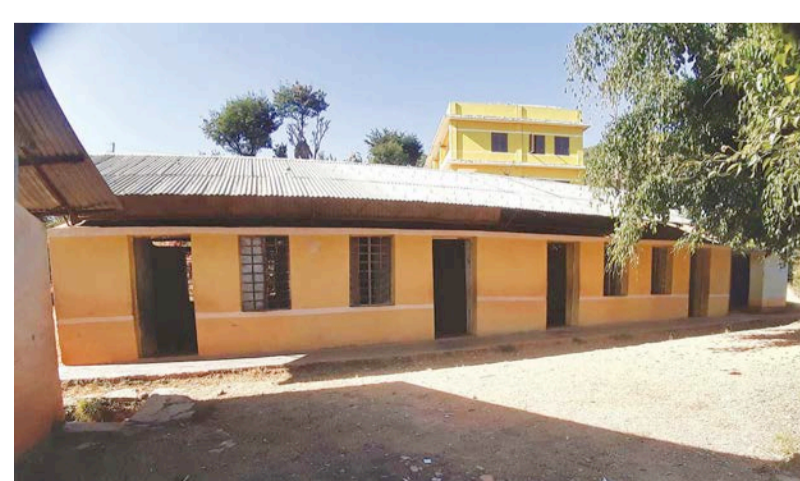
The school building is dilapidated and there are no sufficient desks or even teachers.
