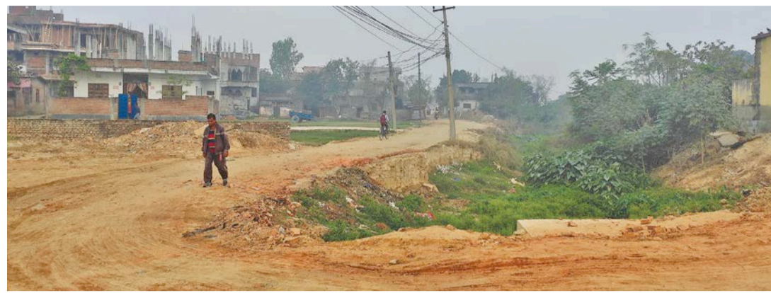
People living in several villages surrounding the Janakpur city have been forced to take lengthy and costly detours after three road sections connecting the city have been disrupted by construction works.
