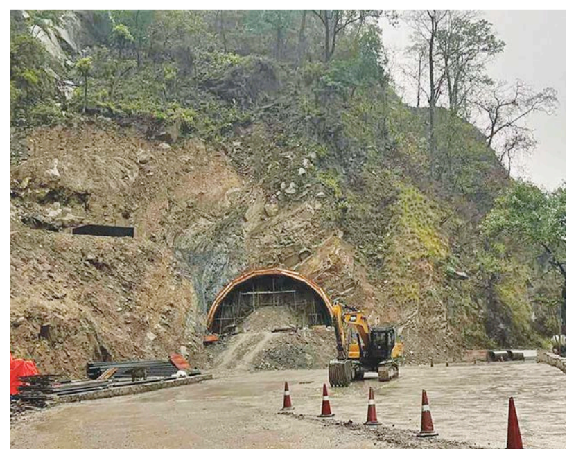
The tunnel starts at Ramapithecus Park on the northern side and ends near Siddha Baba Temple in the south.
