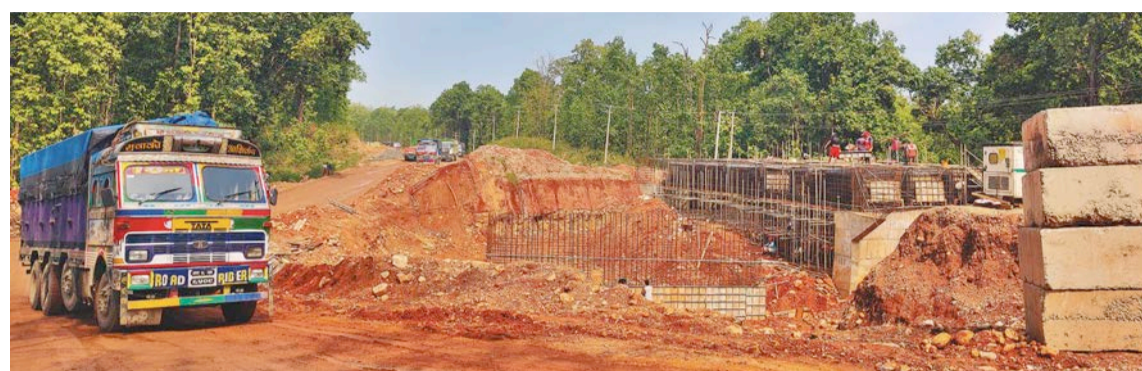
An under-construction Kawasoti section of the East-West Highway in East Nawalparasi, pictured recently. Locals and businesses have long been complaining of dust pollution caused by the construction work.
