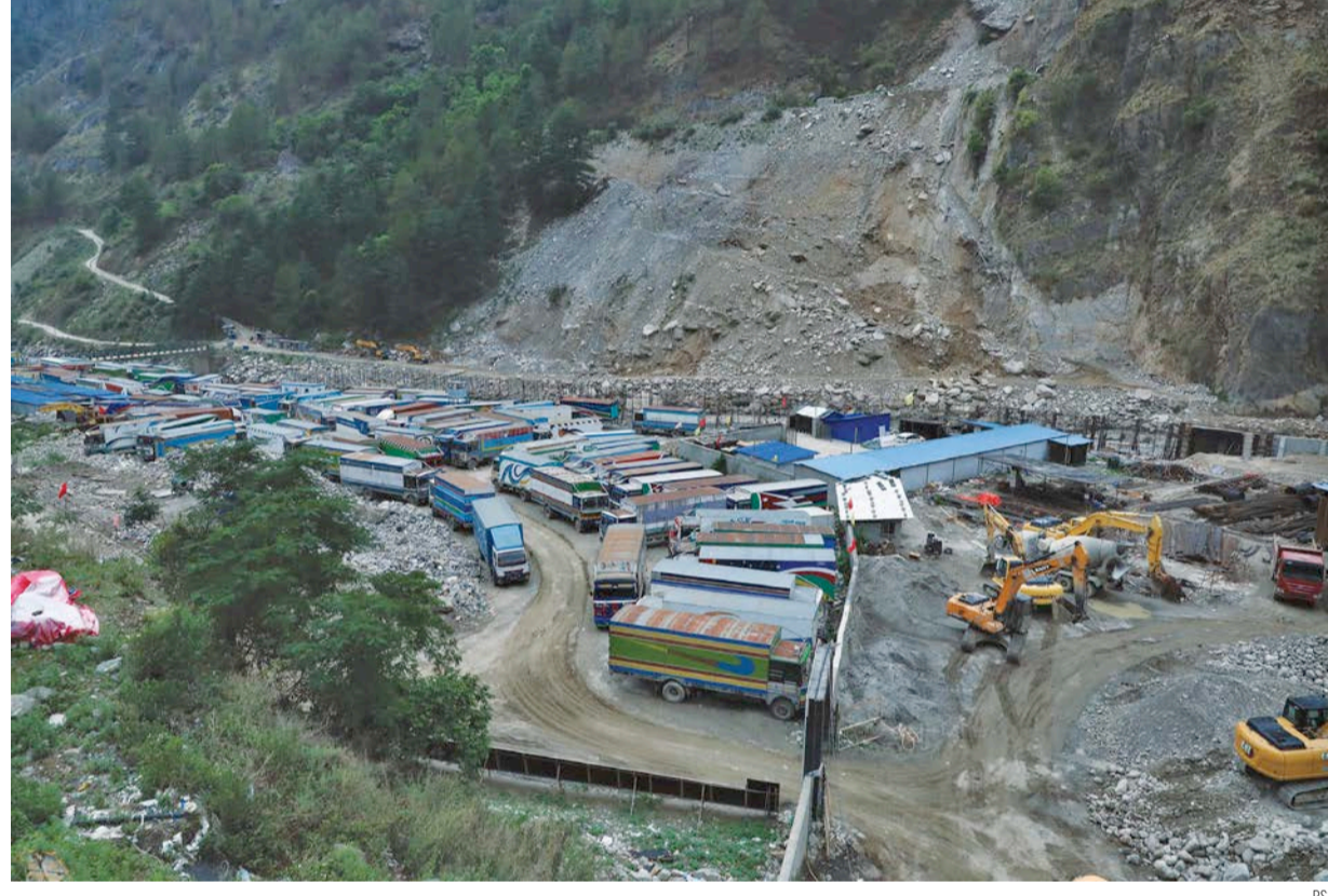
Cargo trucks that entered Nepal from the Kerung checkpoint on the Nepal-China border wait for customs clearance at the dry port in Timure of Syaprubesi of Rasuwa district on Friday. The border point, which was closed since the start of the Covid pandemic, reopened earlier this year.
