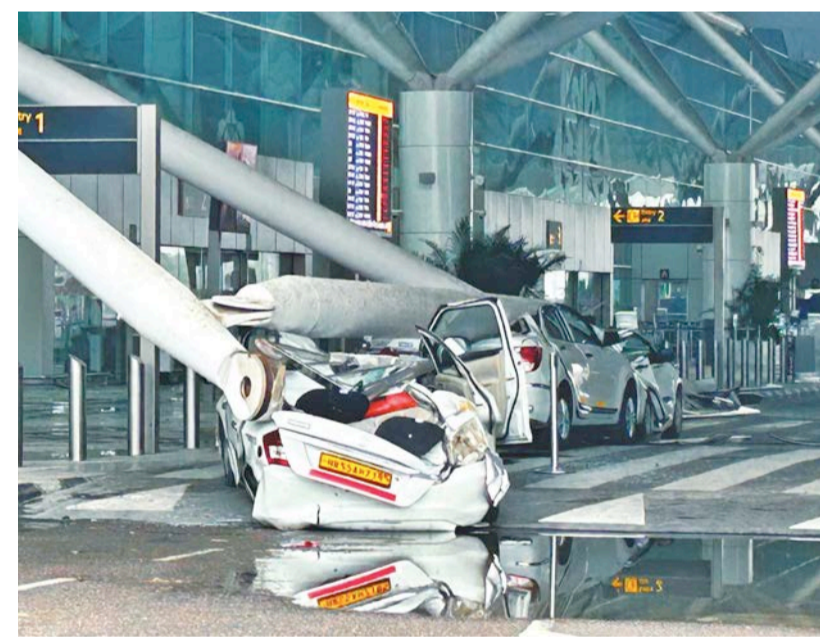
Parked vehicles are damaged by the collapse of a departure terminal canopy at New Delhi's Indira Gandhi International Airport following heavy pre-monsoon rains in New Delhi, on Friday.
