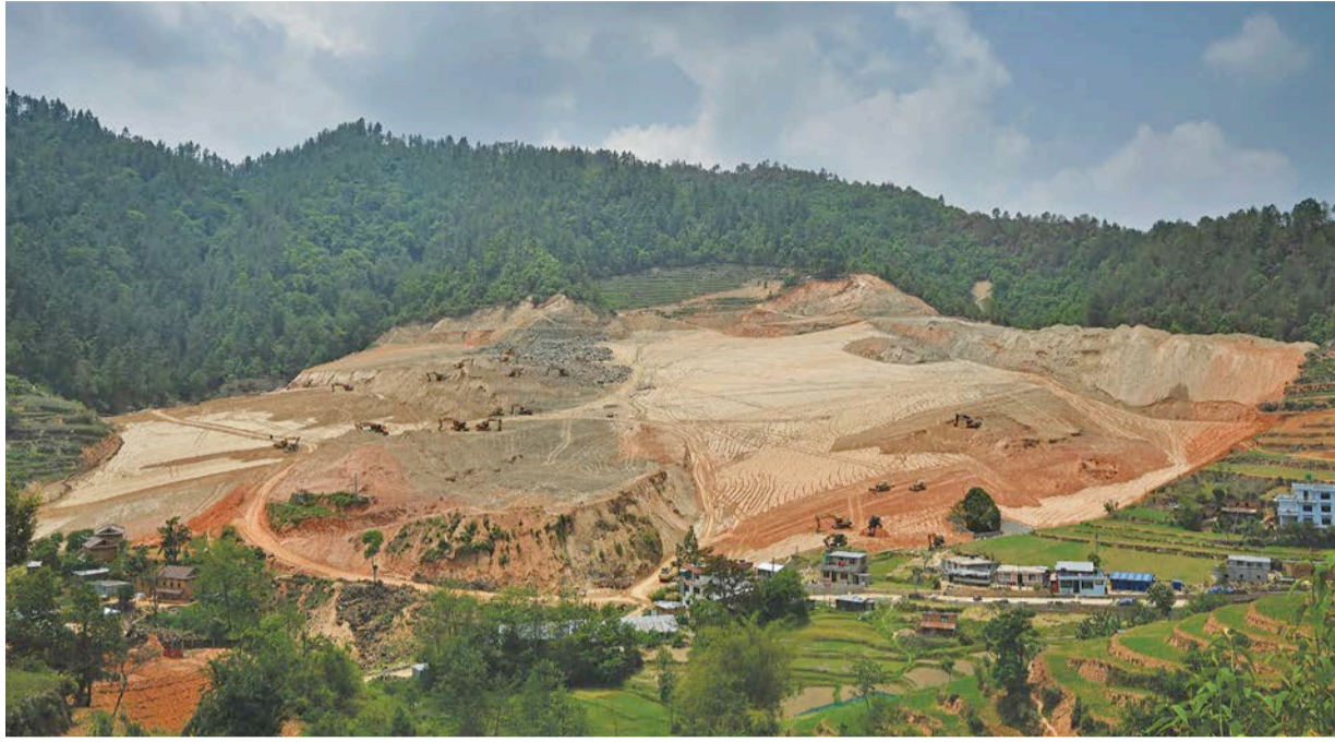
Plotting of forest, farm and public land for housing ongoing at Kakrebari in Suryabinayak-9, Bhaktapur, in this picture taken on Monday. The illegal excavation hasn't stopped despite objections from local residents, local people's representatives and the district administration.
