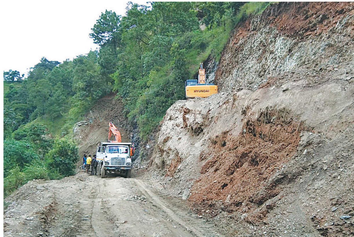
This image shows ongoing road widening work in Khahare of Baglung district along the Mid-Hill Highway.
